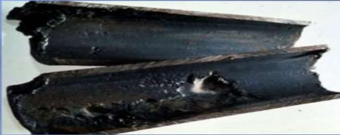
Boiler system tube shows high pH gouging
